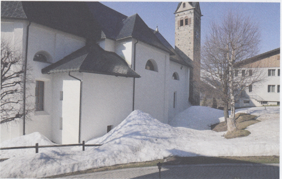
Meters neiv ruschnada dil tetg baselgia che donnegiescha ils mirs.
